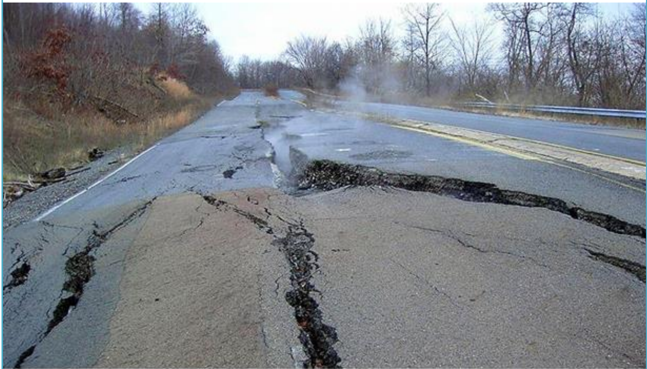
Figure 4.3.12-4: : Centralia Mine Fire damage to PA Rt. 61 (Encyclopedia of Earth, 2006)
